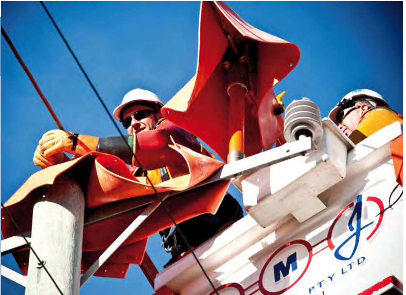
Live-lineworkers John Goodall (front) and Peter Milton upgrade power supplies in Devonport.
